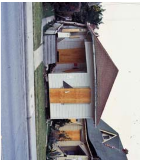
Figure 4 – This Watsonville house shifted off its foundation and fell to the ground during the 1989 Loma Pieta earthquake.
