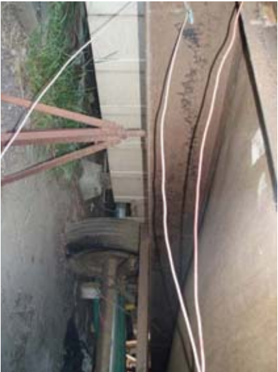
Figure 10 - Typical steel jack support for the small trailer. This type of support does not provide lateral resistance and frequently fails in earthquakes.
