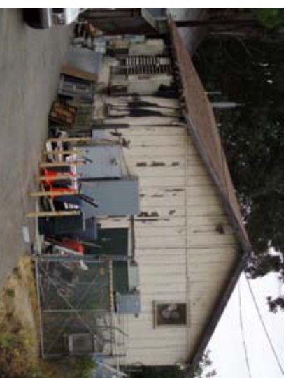
Figure 2 – Wood frame building. This is showing deterioration on its the exterior. The ends of many roof rafters are rotten and the paint is peeling off the siding in many places.
