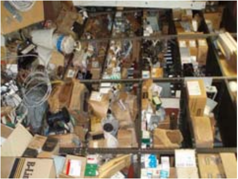
Figure 12 – The contents of these metal storage shelves can topple. Additionally, some shelves in the building are not anchored to the floor and can slide or tip over.
