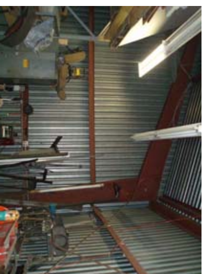
Figure 6– Inside view of the prefab metal building showing a moment frame and rod bracing.
